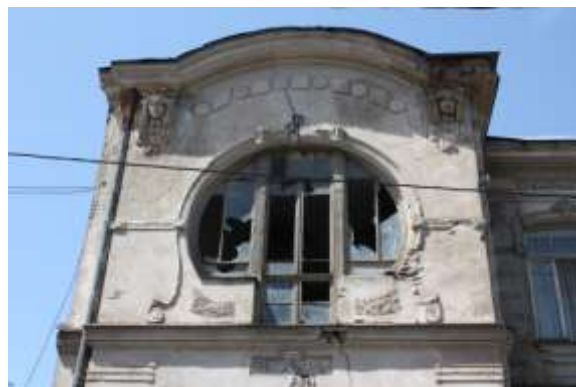
Crumbling Art Nouveau apartment block in Tbilisi, Georgia
