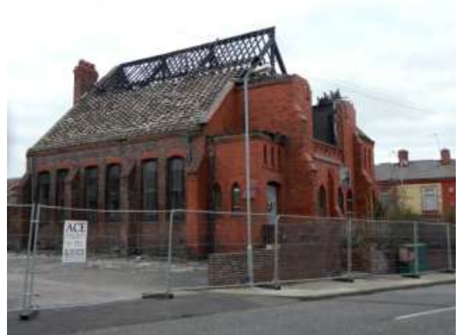
Springwell Chapel, the Klondyke, Bootle, Sefton. Demolition was halted by an injunction from SAVE.
