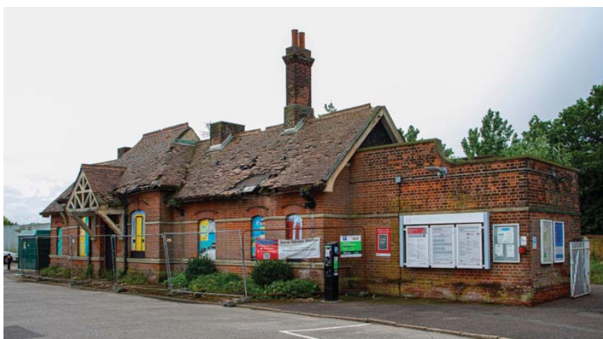
The 1890s station building at Trimley Station in Suffolk which has been similarly left to rot by train operator Greater Anglia, with drone footage in April 2023 revealing the extent of the gaping holes in the building's roof, making the it highly vulnerable to rapid weathering (Credit: Alistair Smith)
